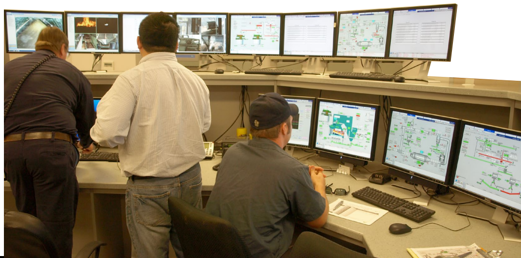
Operator control room for a biomass system
