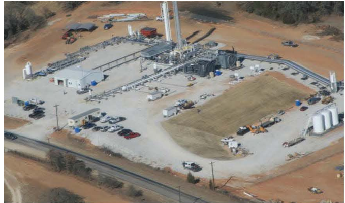
This 200 gal/min amine plant has the thermal fluid heater separated from the rest of the system for safety.
